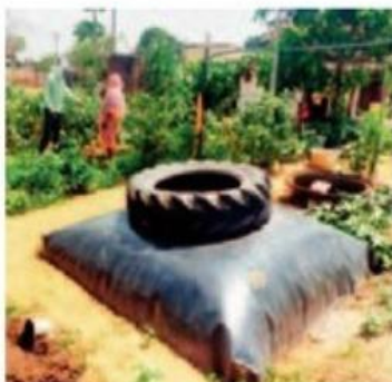
A biogas set installed in one of the villages in Parseoni tehsil of Nagpur district.
